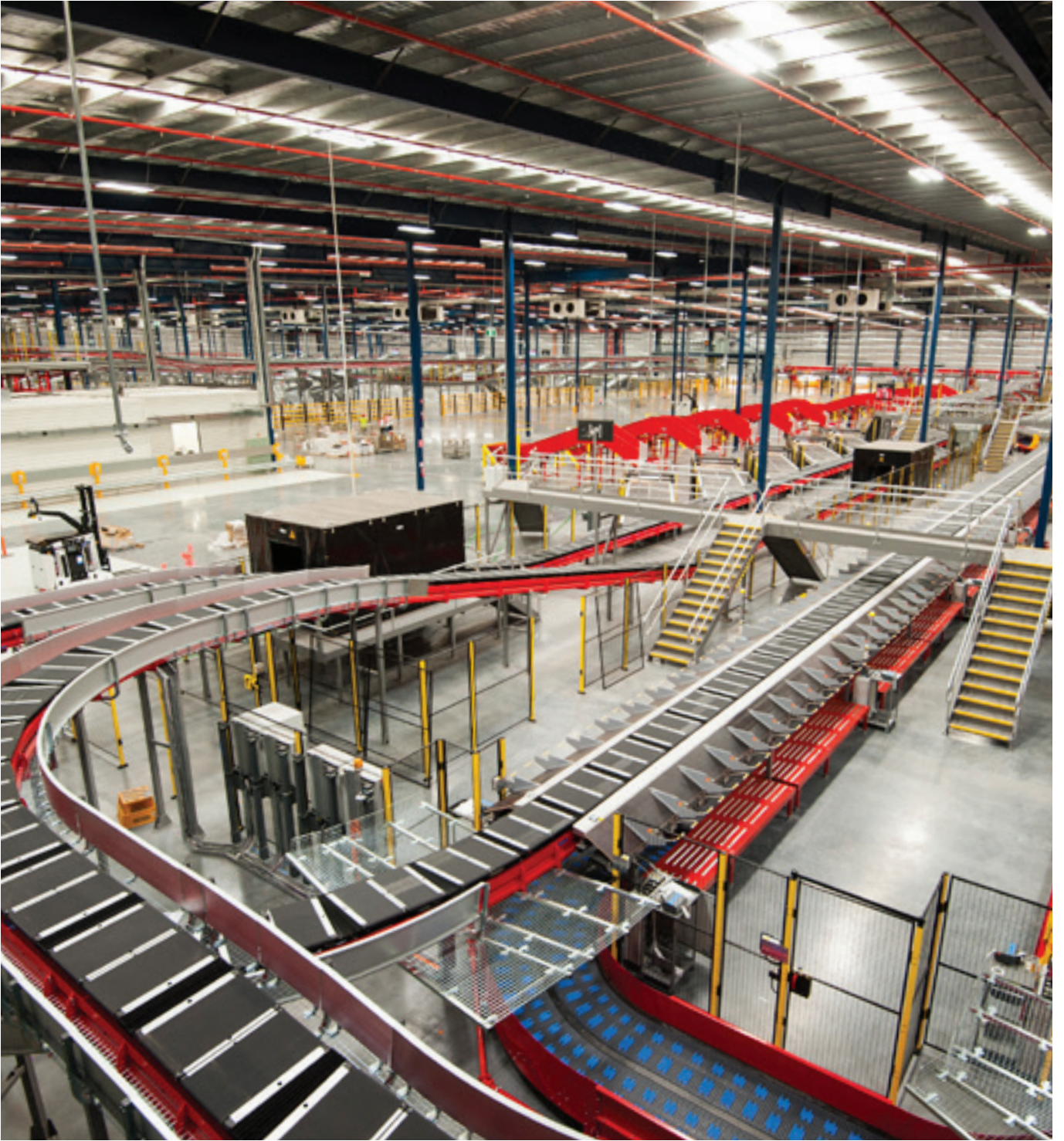
Parcel sorting automation being installed at the new Brisbane Parcels Facility at Redbank.
